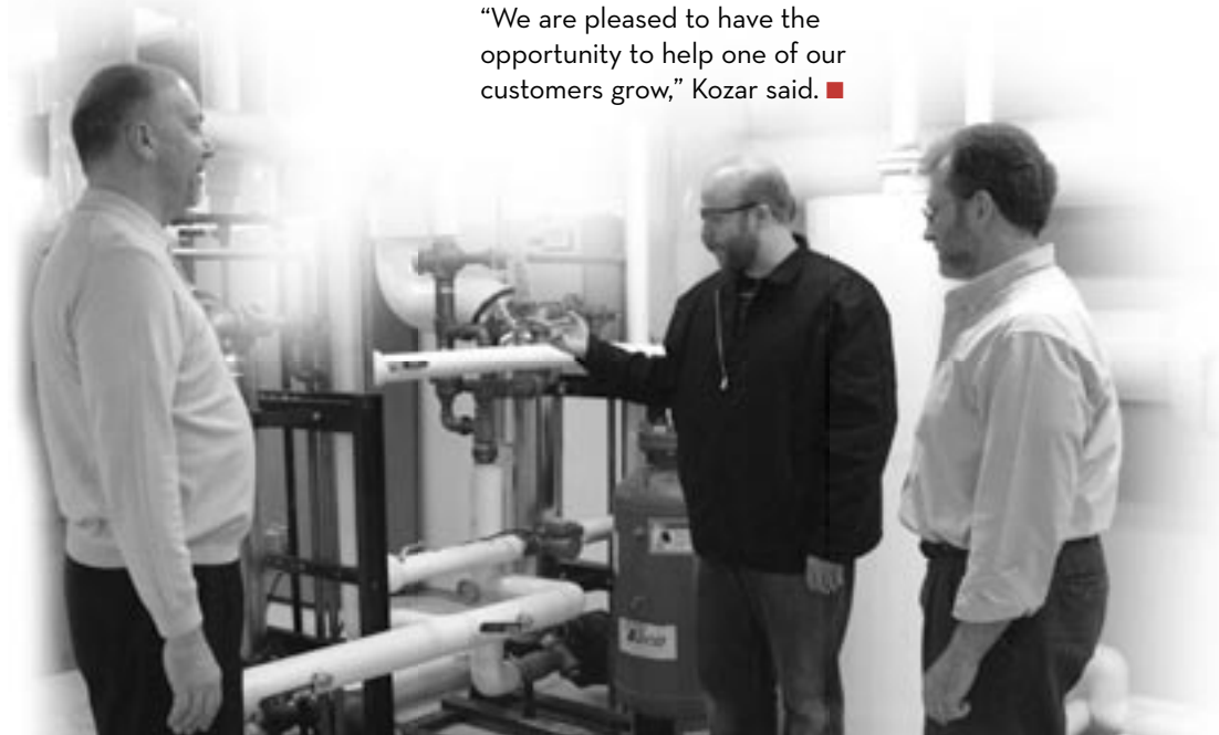
From left: John Kozar; Jeff Smigielski-McHenry, BD facilities engineer; and Lee Bowling examine a section of the company's new steam equipment.
