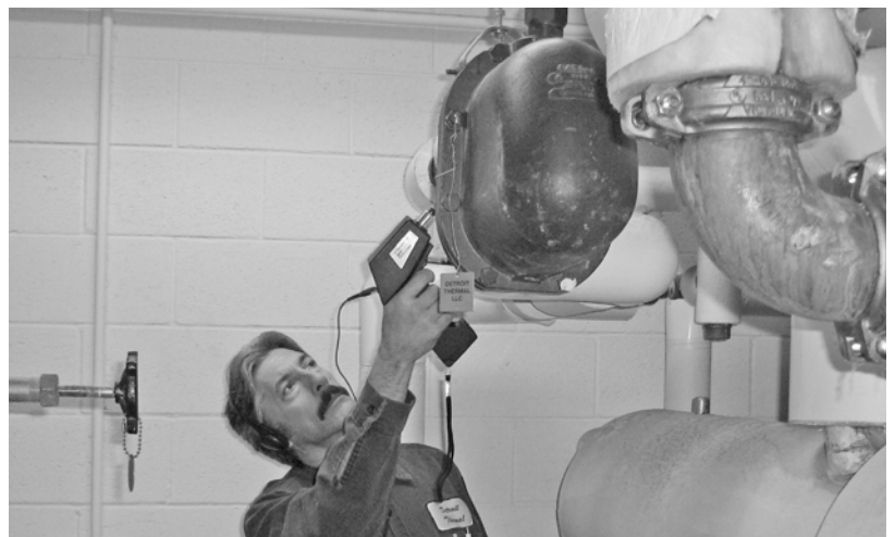
Mike Hoffman, Detroit Thermal customer service technician examines a trap at a customer's site.
